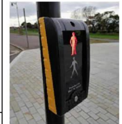
Typical Example of a pedestrian signal push button
